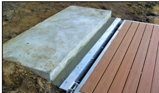
Concrete Angle on New Concrete
